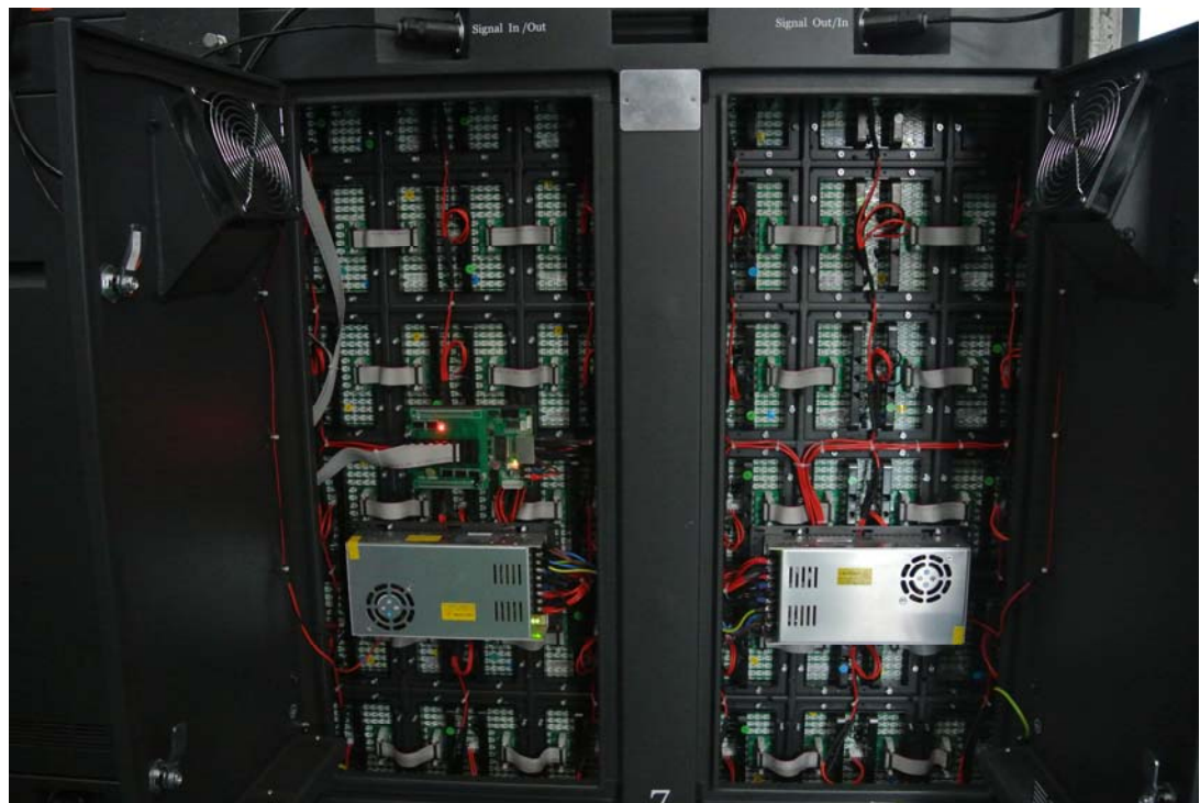
whole look of the inside of a cabinet
