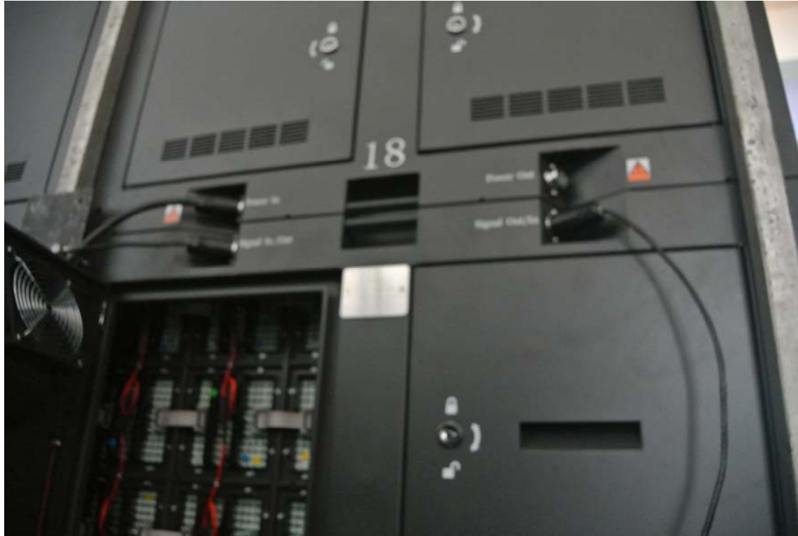
connection between cabinets
