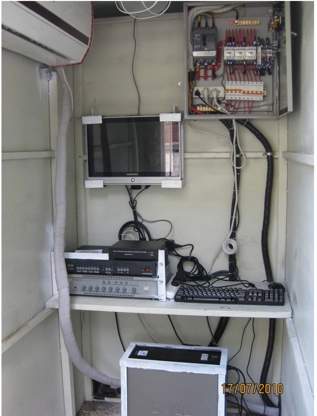
Control room with air conditioner , IPC and power box
